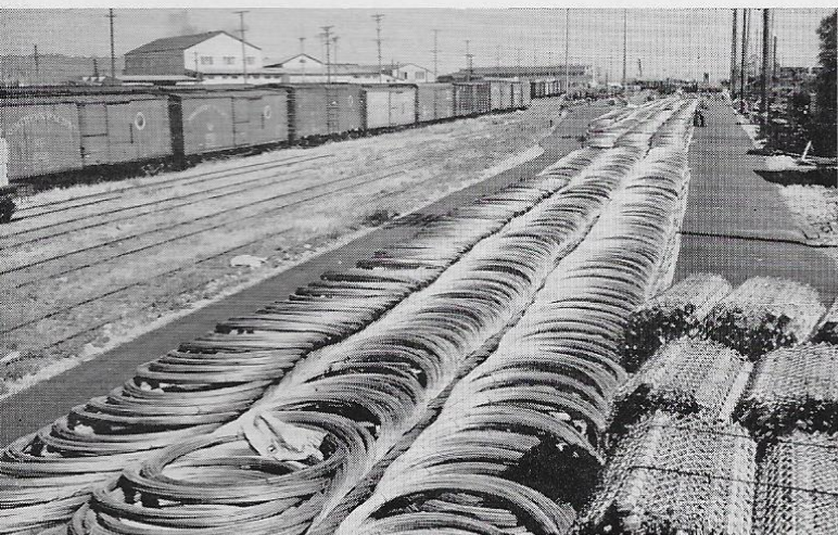
Here is part of nearly 20,000 miles of wire which, when spun into cables, will support the bridge roadway. It was shipped from New Jersey to the West Coast by boat.
