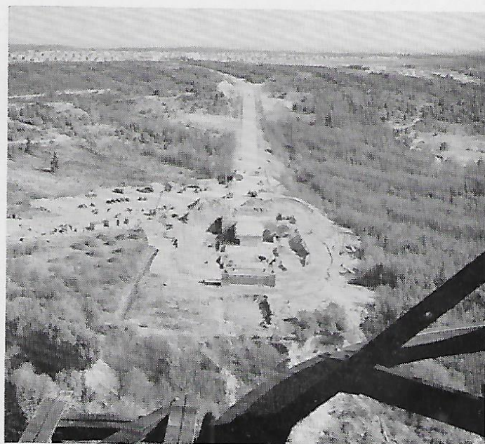
A suspension bridge calls for strong anchor blocks on each bank to grip the main cables. This base on the east shore is shown in the early stages of construction.
